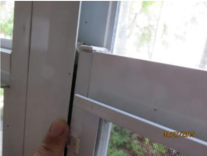
Window repair needed in living room
