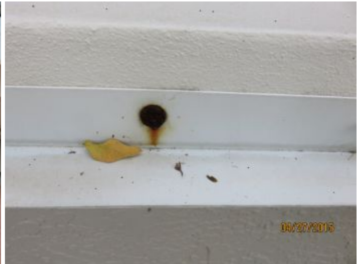
Rusted screws for accordion shutters
