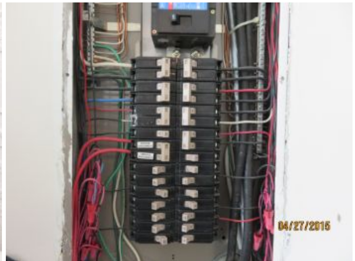
Main distribution panel
