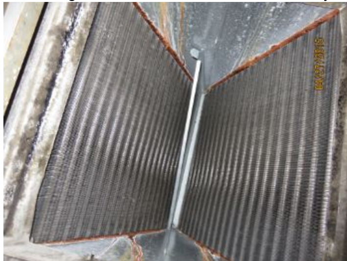
View of coils at air handler
