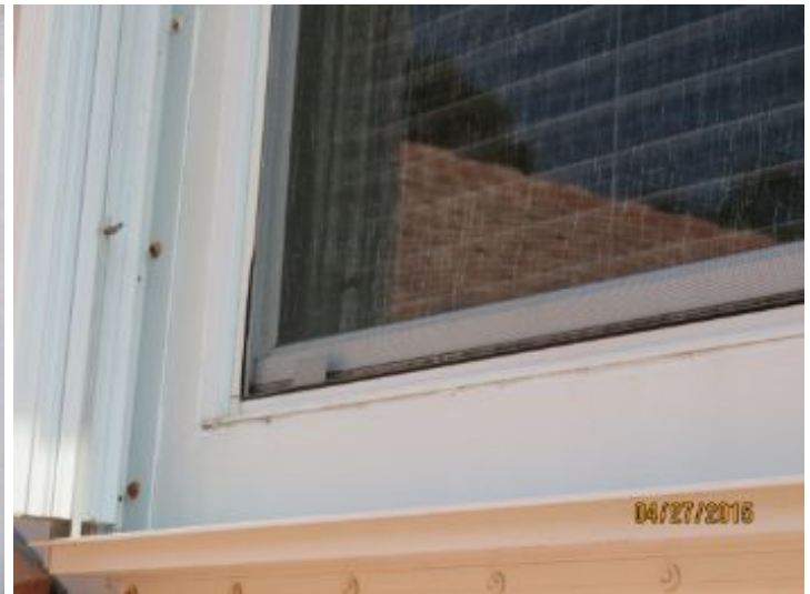
Recommend caulking around all windows
