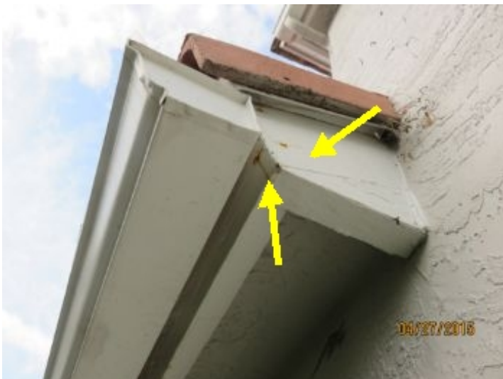
Seal areas of fascia where wood is split
