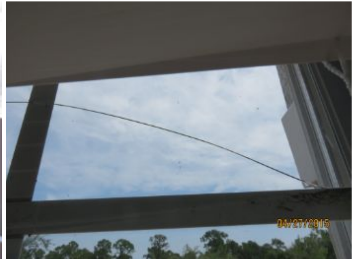
Cracked window in upstairs office
