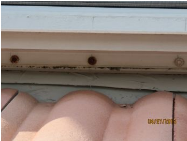
Rusted screws on accordion shutters
