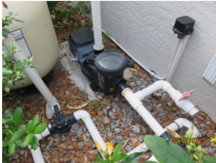
View of pool equipment
