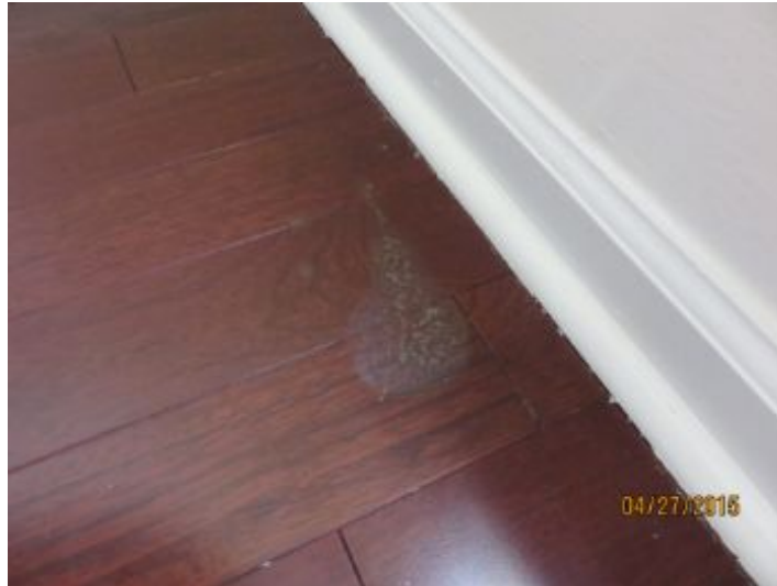
Blemish on wood floor
