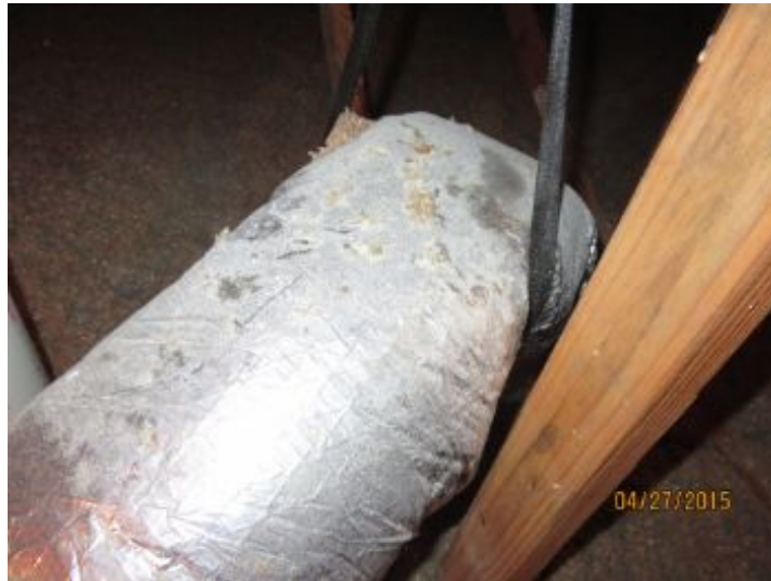
Flexible ducts in attic
