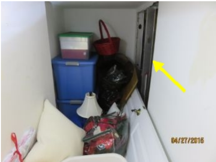
Missing drywall under stairs
