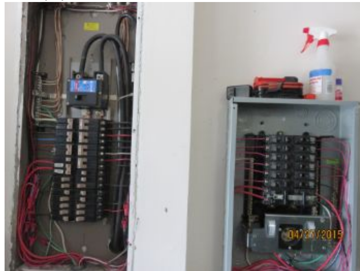
Main and sub panel for generator
