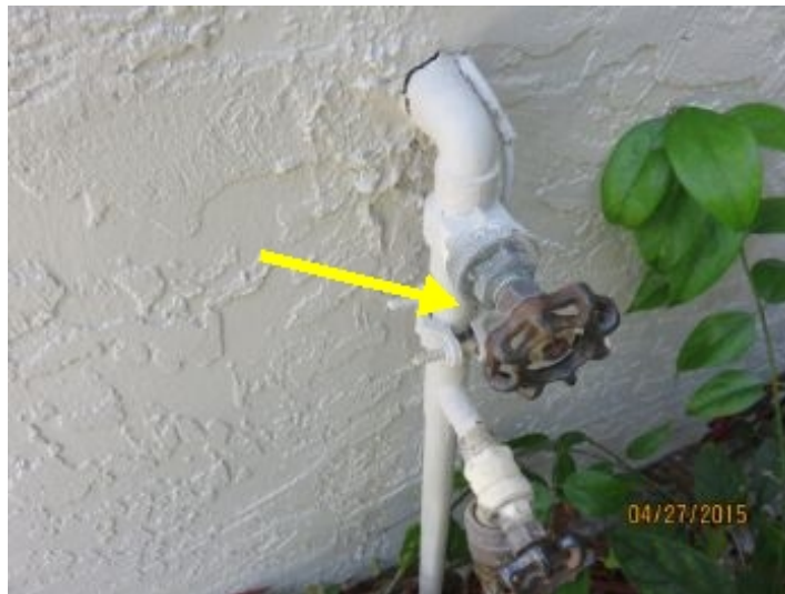
Main shutoff valve
