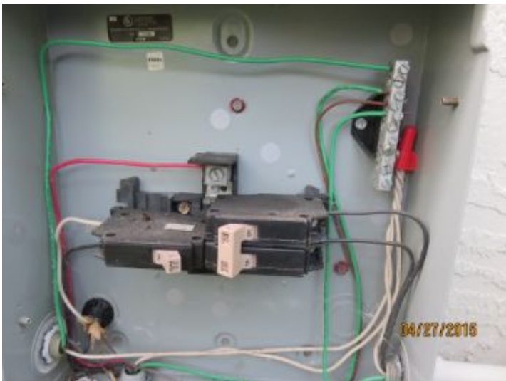
Sub panel at pool equipment
