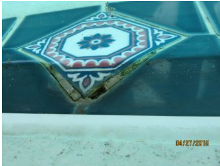
Missing grout and loose tiles
