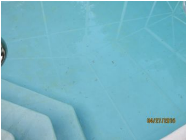
Swimming pool with blemished areas on surface
