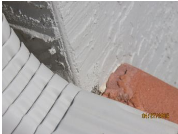
Missing kickout flashing
