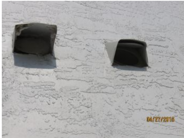
Missing screens for vent fan/dryer vent should be cleaned
