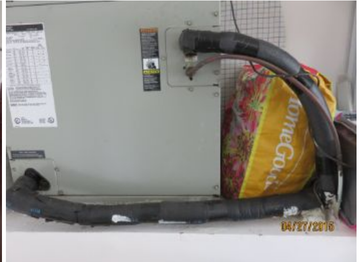
Recommend Safety/Float switch at air handler
